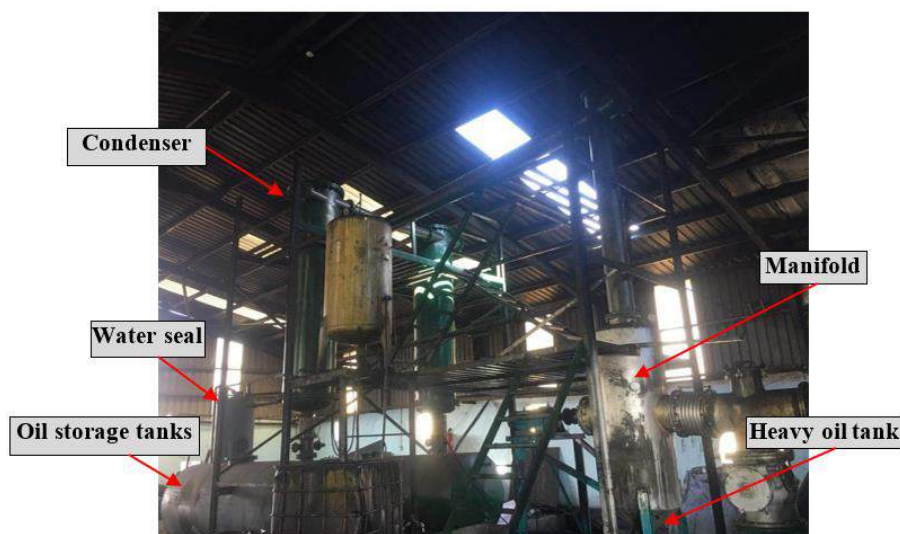
Figure 4. Manifold, heavy oil tank, condenser system, oil storage tanks and water seal.
